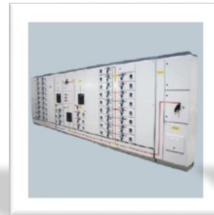
LV + HV Gear Panel
